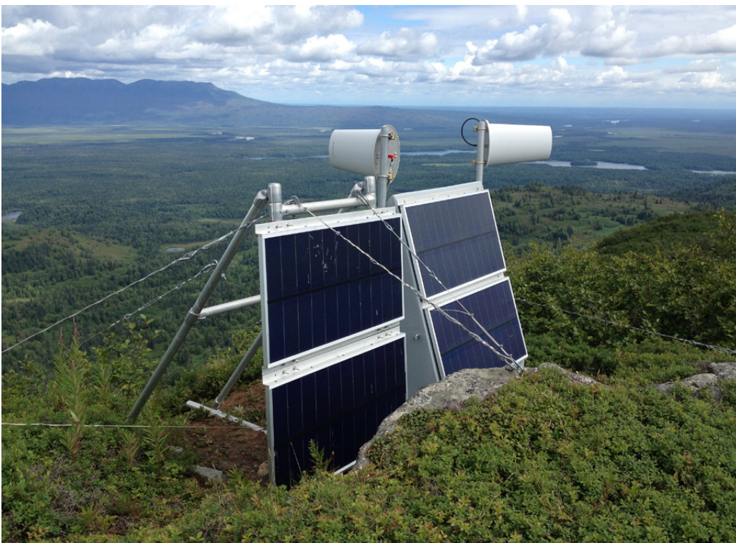
Station AC46 Skwentna lies close to the Iditarod trail in south-central Alaska. The twin radome-shielded antennas relay data from the highest elevation site on the southern edge of Denali National Park, providing important information about the ongoing uplift of the Alaska Range. Photo by Alaska Field Engineer Ellie Boyce.
